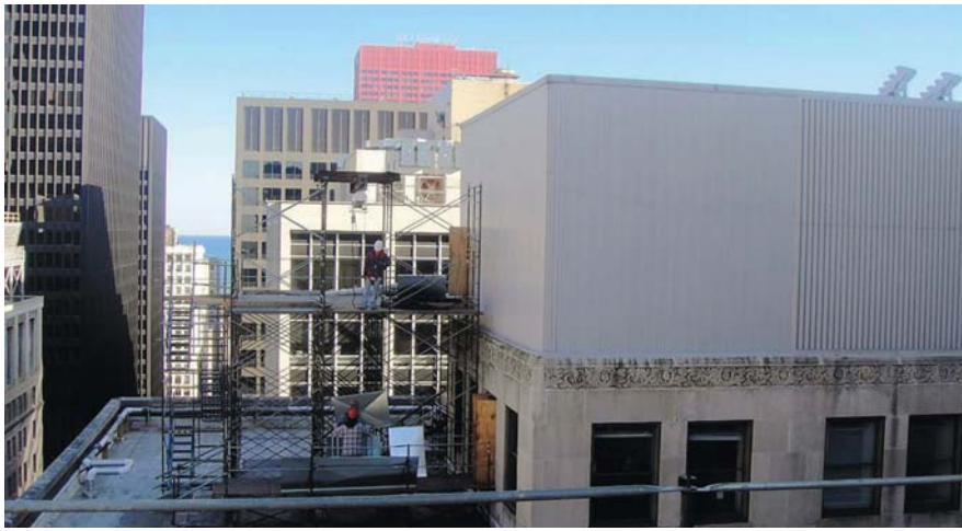
One by one, CPS personnel brought the 72 fan cells up to the 23rd floor using a dolly. The cells were moved outside onto the sub-roof where they were hoisted onto a scaffolding catwalk and moved into the mechanical room on the 24th floor through a temporary hole in the wall.
