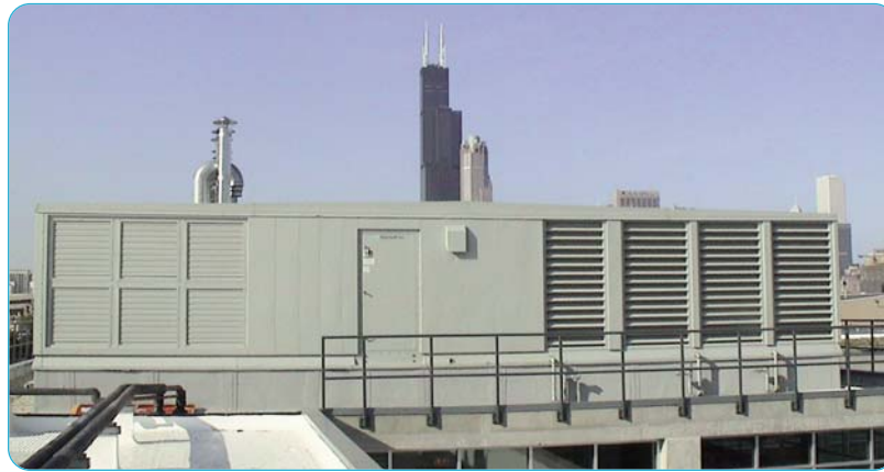
Mammoth® iPEC™ unit supplying HVAC to the Pacific Garden Mission.
